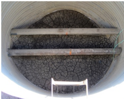
View into bell hole. Virgin pipes are ready for monitoring equipment installation.
